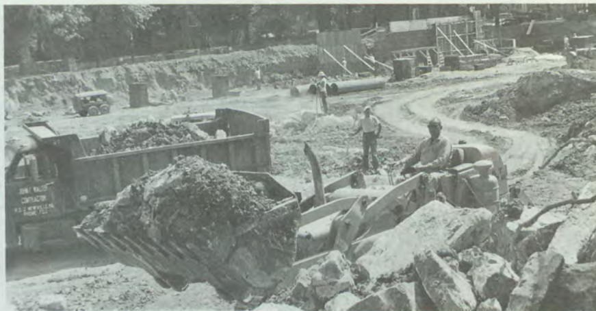
Excavation for the College Center is almost completed and the side walls are under construction. The Center is scheduled for completion in September of 1964.
