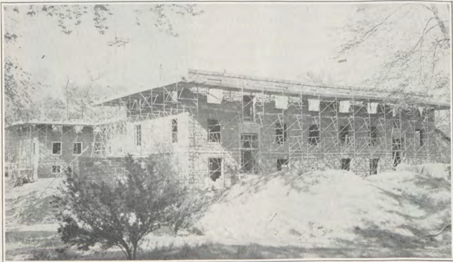
Come Back to Commencement and see Morgan Hall, the new dormitory for men now being built on the Benjamin Rush Campus. The above photograph was taken on May 1, 1955. Builders plan to complete the structure for use next September.
