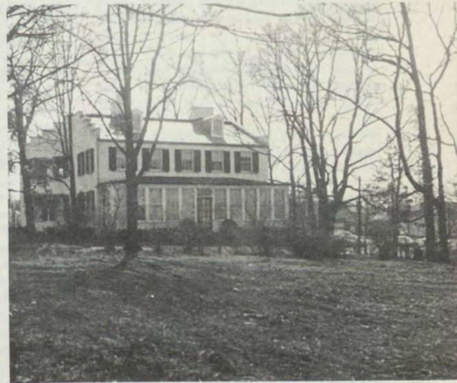
The razing of Metzger Hall is completed as shown by this view of the property taken from the former location of the front porch. In the background is the Hays House.
