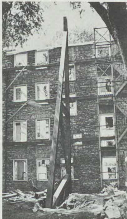
Collapsed East College before reconstruction as The Bernard Center for the Humanities, 1968-70.
